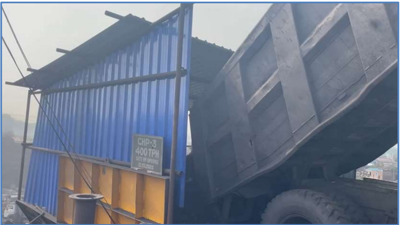
Picture 7 – Enclosed Coal Handling Plant
