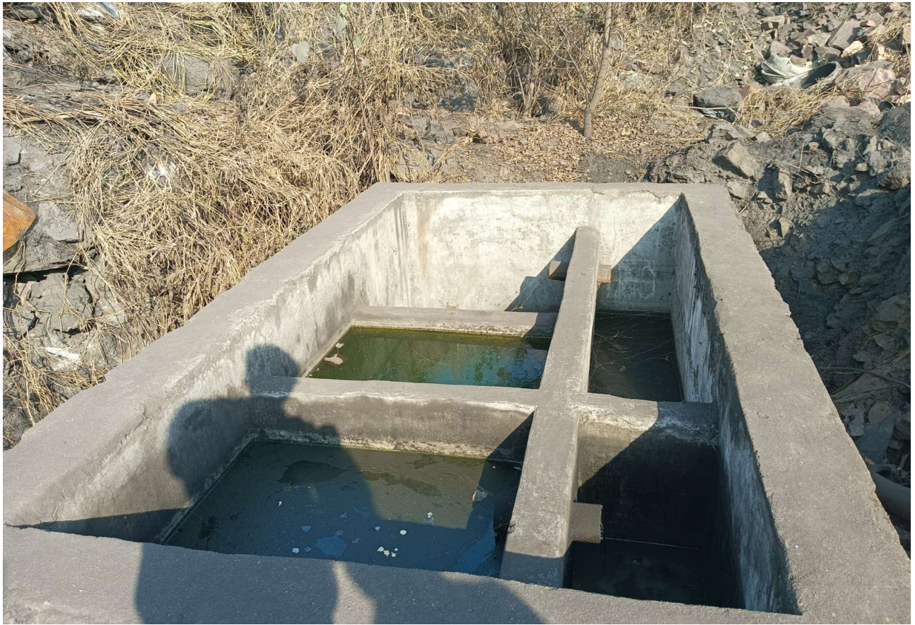
Picture 10 – Oil & Grease Trap
